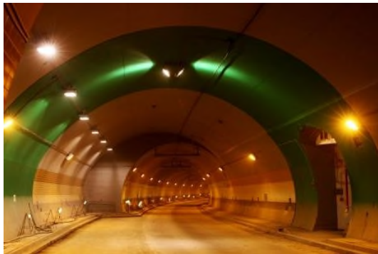
Emergency stopping bay in the Bubeneč mined tunnel (photo Jakub Karlicek)
