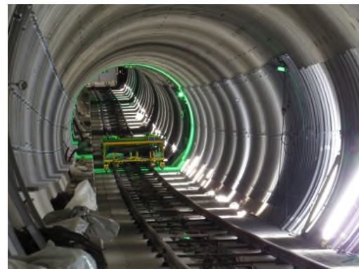
Connection of the left-hand track to the existing metro line (photo Jiri Junek)
